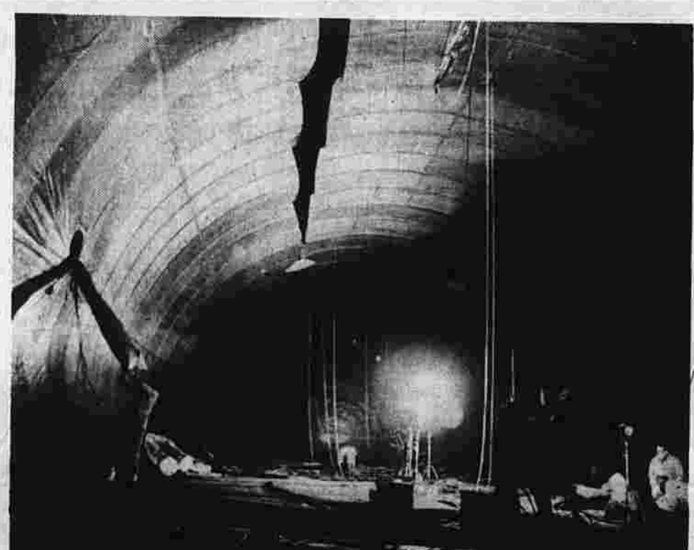
In the America's cave-like interior skilled riggers install cables which will secure the gondola to the envelope.
